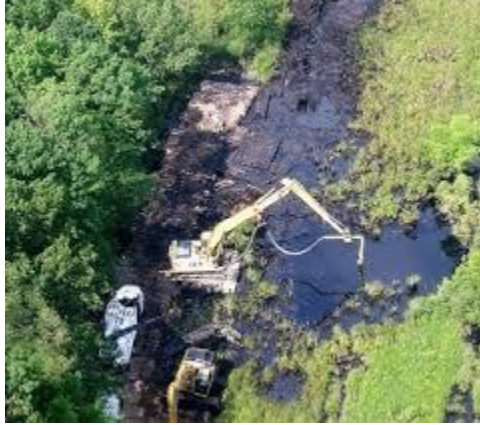
Figure 8.8 Response operations near the source of the spill on Talmadge Creek. Image from US EPA.
